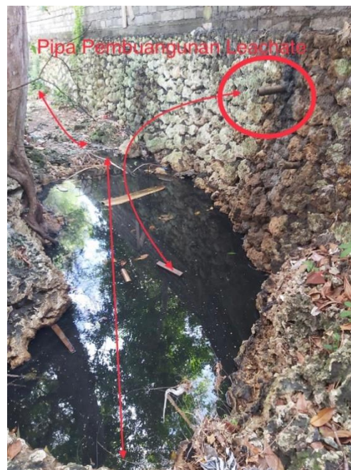
Figure 7. Leachate flowing to community's property January 2023
