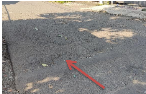
Figure 9. Peeling of the Surface Layer (Source: Research Results)
