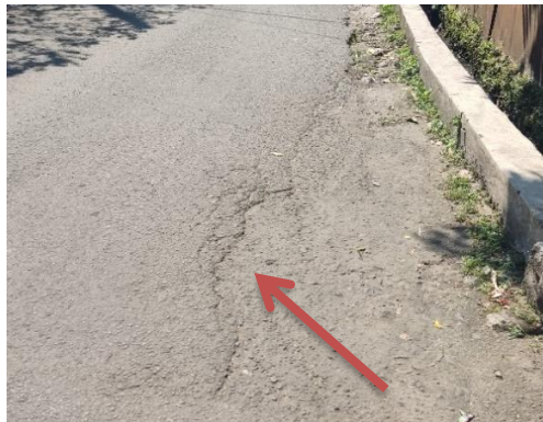
Figure 8. Side Cracks (Source: Research Results)
