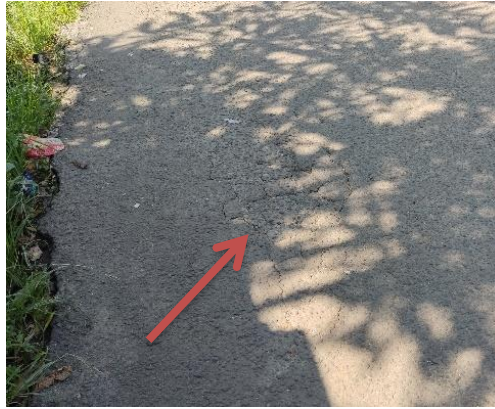
Figure 6. Cracking (Source: Research Results)
