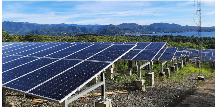
Figure 2. Solar Panel in Indonesia
