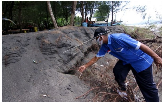
Figure 8. Damage to Cemara Beach due to Abrasion
