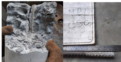
Figure 7. Steel bar condition
