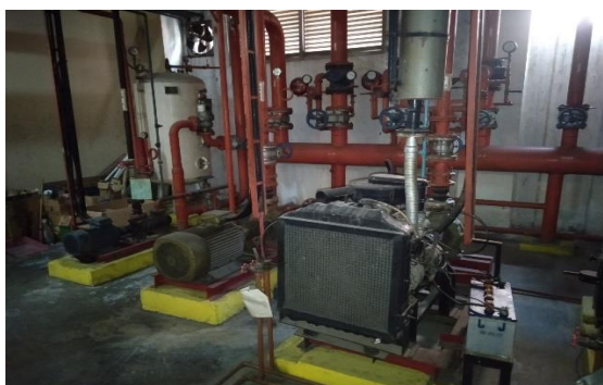
Figure 4. Hydrant Drive Source and Sprinkler
