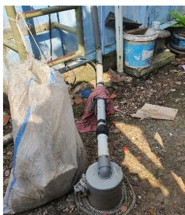
Figure 3. Piped water to the reservoir (Observation, 2021)
