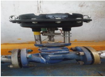
Gambar 2.8 Control Valve Blowdown Boiler
