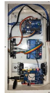
b. Box panel ruangan
