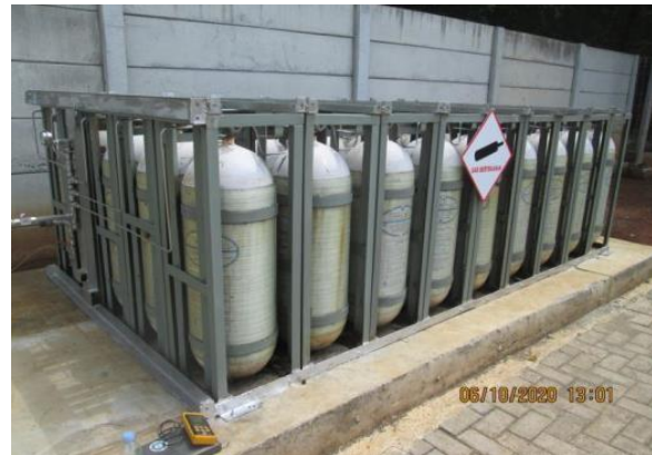
Gambar 2. CNG Buffer Storage Tank
