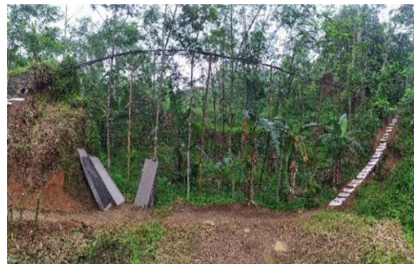
Figure 1 Channel damage condition
